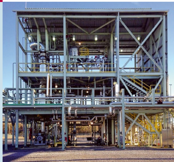
Continuous HHCR Plant, US
